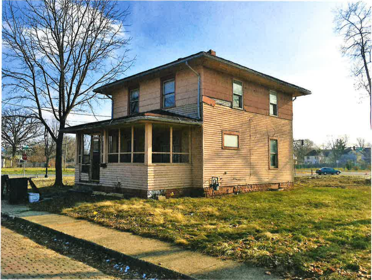
618 Marion Street Tax ID 018-1055-2355 Vacant, Abandoned, Structurally Deteriorating House See Attached Photos
