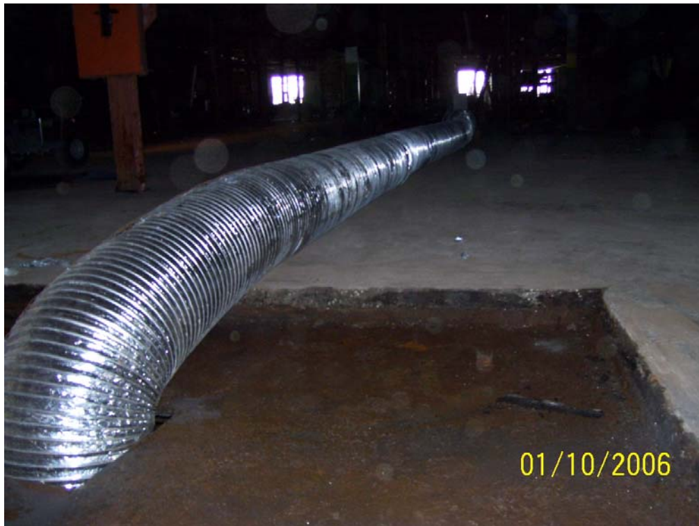
Site: South Bend Lathe Removal Photo Number: 7 Direction: North Subject: Exhaust vent for west transformer room
