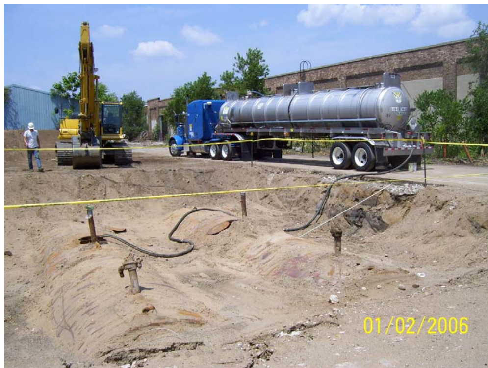
Site: South Bend Lathe Removal Photo Number: 8 Direction: West-Northwest Subject: Contents of the south 20,000-gallon USTs being transferred to a tanker for transport
