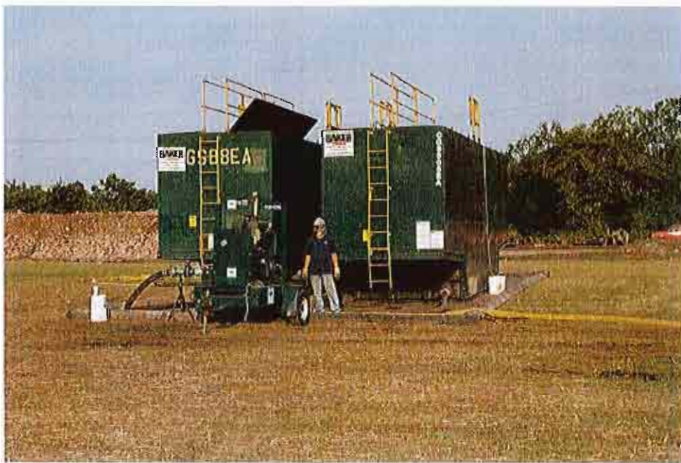
No. 2 – Two 21,000-gallon portable water tanks used for mixing of permanganate solution.
