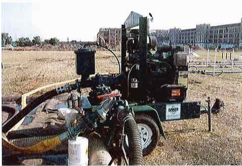
No. 3 – Diesel pump (900 gpm) used for mixing and injecting the permanganate solution.
