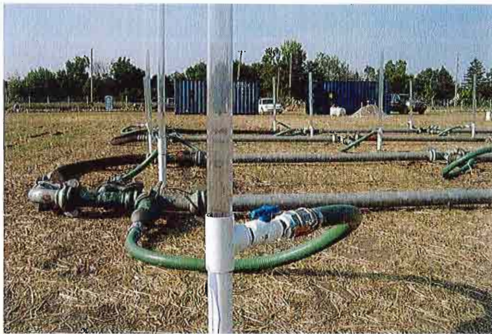
No. 5 – This close up image illustrates a typical injection well head and its control valve.
