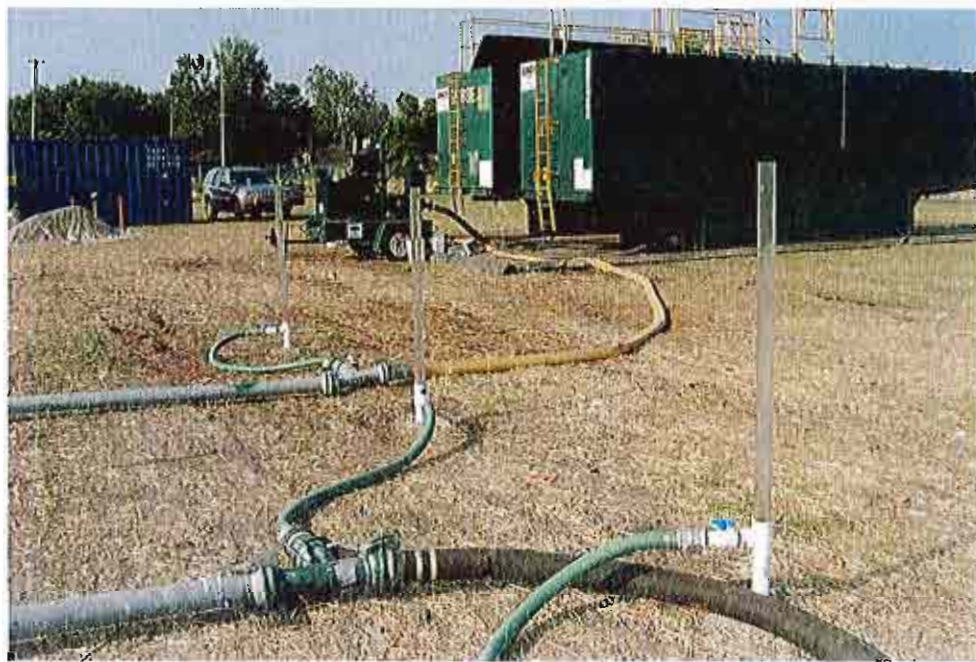
No. 6 – This photograph illustrates the main feed from the mixing/injection pump to the well field distribution system.
