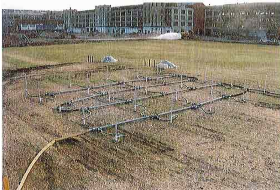
No. 4 – This is an overview of the permanganate injection well field looking to the northeast. The injection well at the far left is IW-A1. The well at the top is IW-E1. The well furthest right is IW-E5. The well at the bottom of the photograph is IW-A5.
