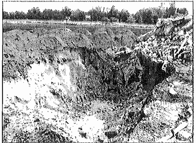
Photograph No. 8: View of Empty Excavation Pit, with Backfill piles in Background (From North-West)
